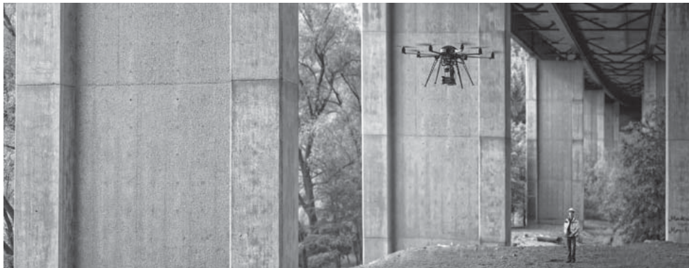
The high-tech miniature aircraft scans building structures in just a few hours. (© Uwe Bellhäuser) | Picture in color and printing quality: www.fraunhofer.de/press
