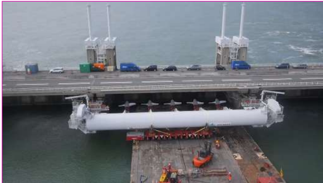
1.25MW dam-integrated array of 5 turbines Eastern Scheldt Storm surge barrier
