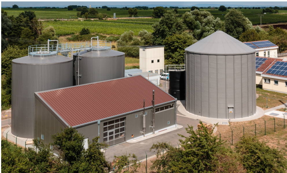
The two-stage high-load anaerobic digestion system in Edenkoben allows the wastewater treatment plant to cope with a higher effluent load during the wine harvest. © Verbandsgemeindewerke Edenkoben | Picture in color and printing quality: www.fraunhofer.de/en/press
