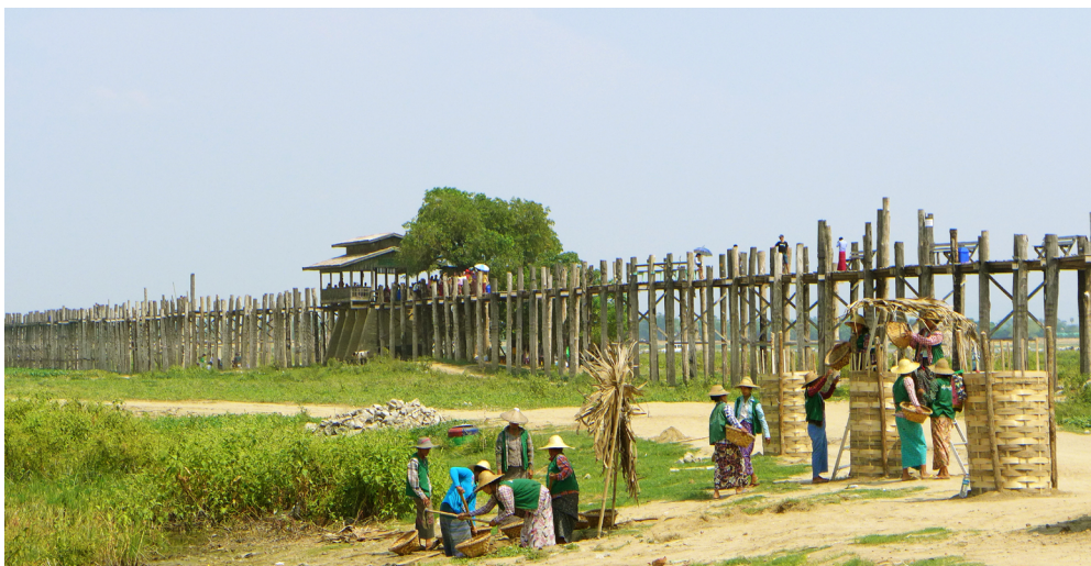
Many of the over 150-year-old posts that support the deck of the world's longest teak bridge need to be replaced. The recovered wood will be reused to make handrails or rest benches along the footbridge. © Fraunhofer WKI/Peter Meinlschmidt | Picture in color and printing quality: www.fraunhofer.de/en/press
