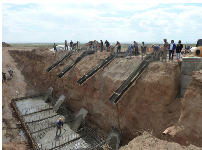
Construction of a water treatment plant in Teshig Soum, Bulgan Province © Fraunhofer IOSB-AST | Picture in color and printing quality: www.fraunhofer.de/en/press
