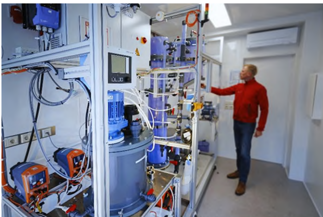
Fig. 1 Test container at the joint water treatment plant in Bitterfeld-Wolfen. Here, new water technologies are tested under practical conditions in order to recover energy and valuable raw materials from chemical process waters.
