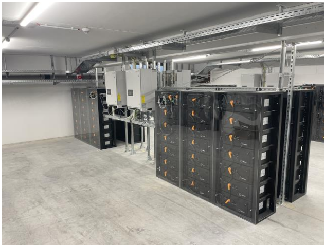
Fig. 2 The modular battery storage units in the Haid project are charged using photo-voltaics and integrated into the energy management system. The system is able to limit any load peaks that might occur by throttling the batteries' charging capacity.
