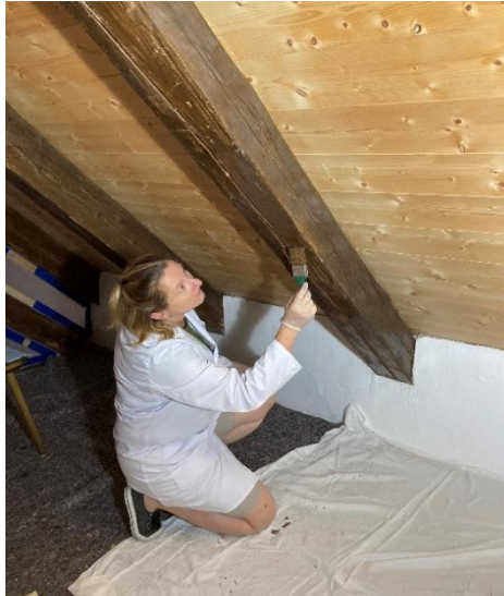
Fig. 2 Dr. Burdack-Freitag of Fraunhofer IBP applies the cyclodextrine formula to a contaminated wooden beam.
