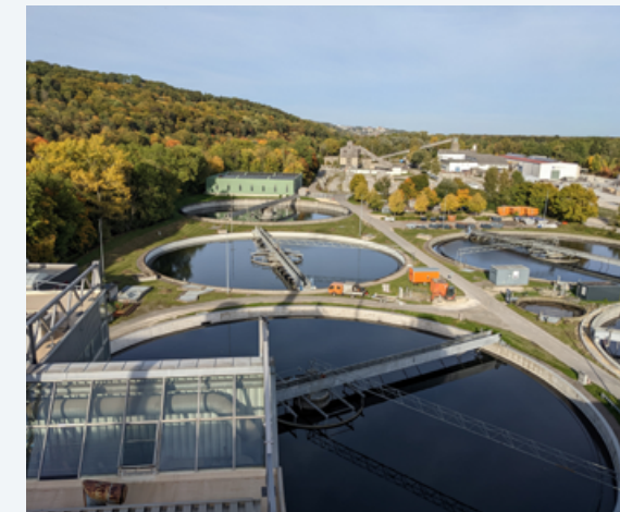
Clarifier at the Ulm-Steinhäule wastewater treatment plant
