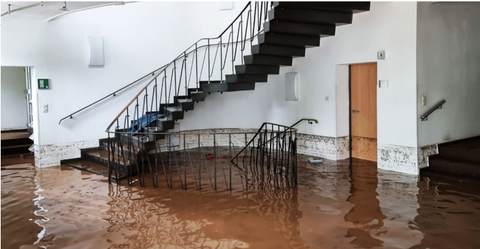
Fraunhofer INT was also directly affected by the catastrophic flooding in the Ahr Valley in 2021. Photo: Fraunhofer INT
