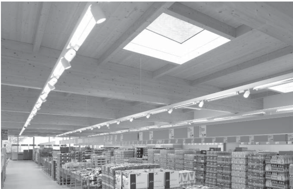
Skylights in the roof reduce power requirements for lighting. (© Ralph Kensmann, StartDesign GmbH) | Picture in color and printing quality: www.fraunhofer.de/press
