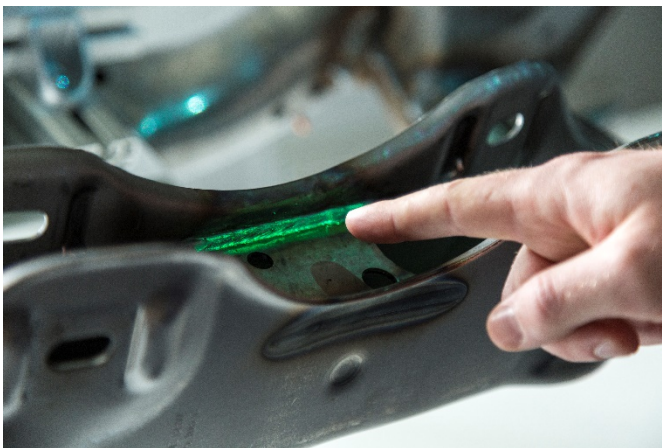
Picture 2: The position of weld seam defects identified by the user can be determined by a combination of finger tracking and 3D seam tracking, and precisely documented.
