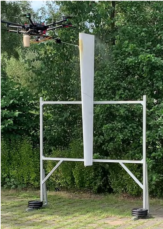
Fig. 1 Coating drone during a spray test: The coating material is applied by the drone via a lance.
