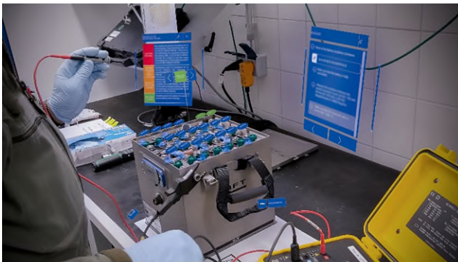
Fig. 3 Carrying out a battery test with guided resistance measurement in the workshop.
