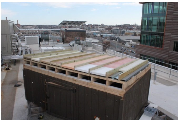
Phenolic foam test hut on the rooftop of Fraunhofer CSE's Boston office building. © Fraunhofer USA Center for Sustainable Energy Systems CSE
